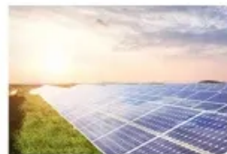
Energy Storage System
